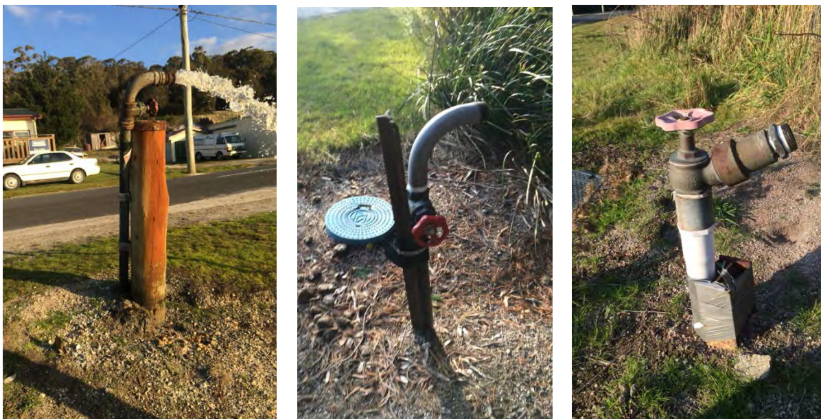
Figure 2. Pioneer town hydrants
