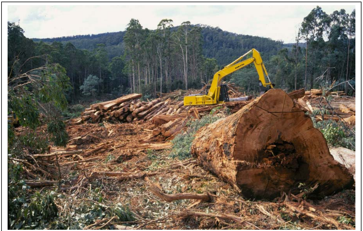
A photo of Gunns 'Larcombes' block during conversion, looking down the slope showing the steepness with the logged out white gum forest in the background, below the logging landing and machine.
