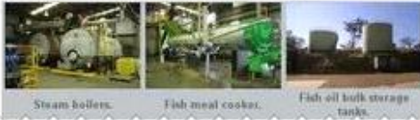
Steam boilers. Fish meal cooker. Fish oil bulk storage tanks.
