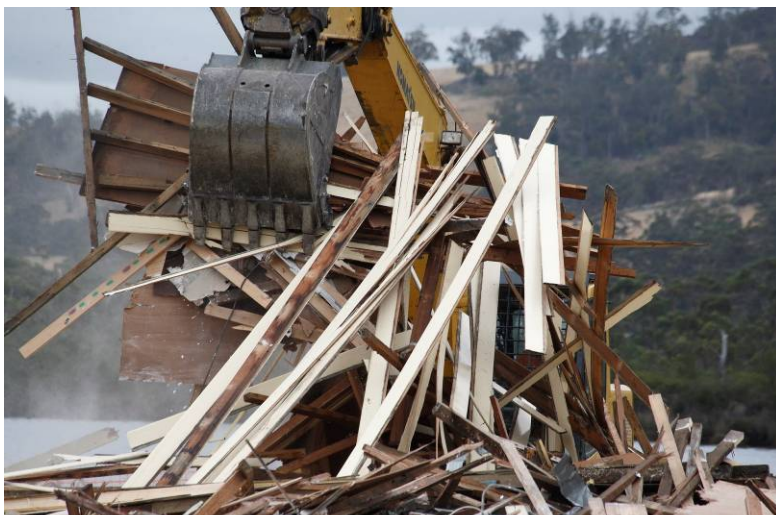
Good roofing iron, wonderfully preserved weather boards, tongue and groove flooring – all trashed.
